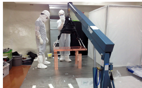
Student Clint Wiseman (left) and Assistant Professor Vincente Guiseppe (right) directing the initial construction of copper shield for the Majorana Demonstrator neutrinoless double-beta decay experiment. The cleanroom laboratory is located 4950 feet beneath the Black Hills of Western South Dakota. Guiseppe manages the design and construction of the experiment's ultra-low background shield.
